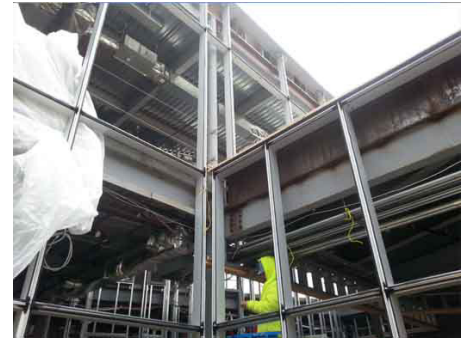
Figure H: Right and below: Structural members of the glazing system are engineered to support the cladding material.
