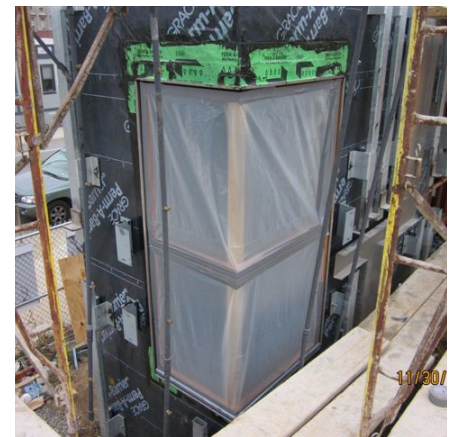
Mockup testing prior to cladding installation isolates the window to verify the integrity of the window-to-wall transition.
