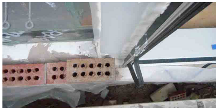
FIGURE 2: From top: Shop drawing submission for typical glazing system jamb; comments to address thermal control as a fire requirement; condition before installation of insulation and fire stopping
