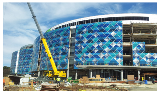
Above top: stick-built curtain wall on the Independence Blue Cross Building (image courtesy Paul Rabinowitz Glass Co., Inc.); above bottom: installation of unitized curtain wall on Nemours Alfred I. DuPont Hospital for Children (image courtesy R.A. Kennedy & Sons, Inc.)
