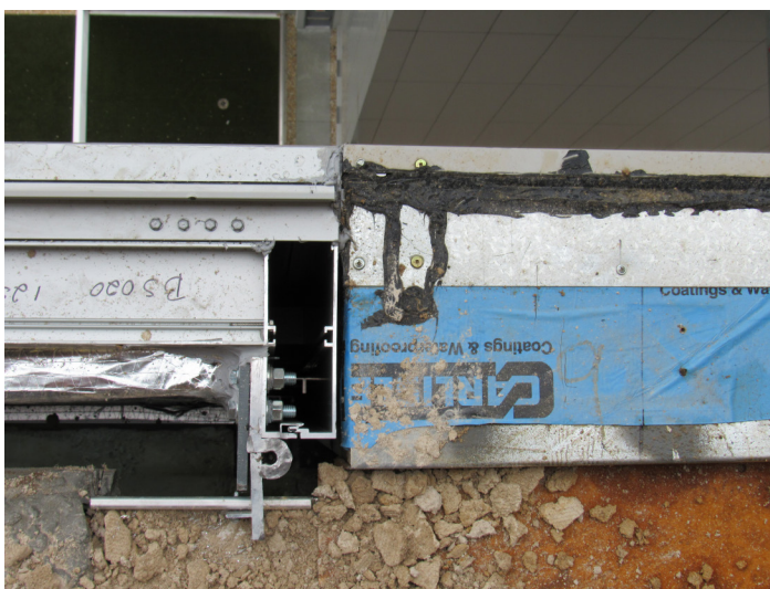
Conflict between unitized curtain wall and prefabricated wall panel: no space was left to install a proper sealant joint between systems.
