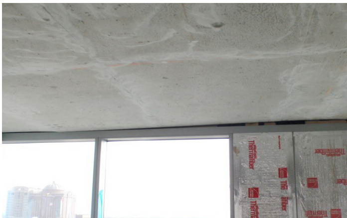
Undulations inherent to precast concrete plank construction create joints that vary in width at fenestration perimeters.
