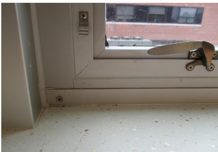
Example of condensation on interior of fenestration system due to improper system selection and/or detailing.
