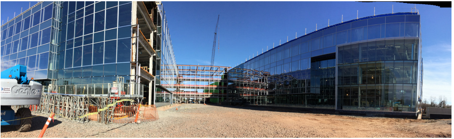
Above: two of the four buildings nearing completion; west atrium wall in background (all photos courtesy National Glass & Metal Co.,Inc.)
