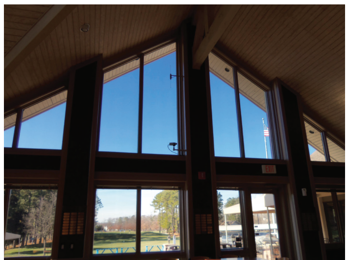
From top: Eastern Solar glaziers applying film at Cooper University Hospital, Voorhees, N.J. (note the privacy film on the left panels); H&M store, Atlantic City, N.J., with solar film applied; Blue Heron Pines Golf Club, Galloway, N.J., with film applied
