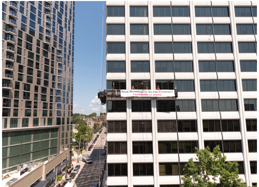
Window replacement underway at 3535 Market (all photos © Paul Rabinowitz Glass Co., Inc.)
