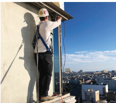
Matt on the job at the South Jersey Gas building in Atlantic City, NJ
