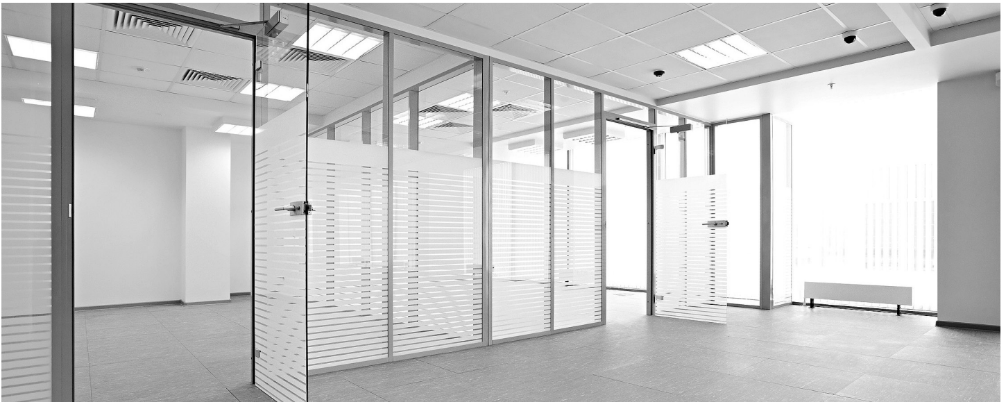
Above: Interior glazing offers natural light, views, acoustic privacy, and a clean, contemporary appearance.
