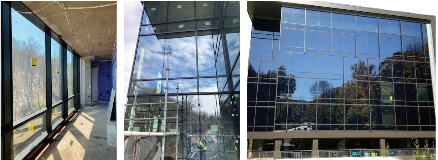
Above: SageGlass dynamic glass installation at 1K1 (images courtesy R.A. Kennedy & Sons)
